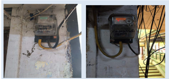
Fig. 13 PROVISION OF EARTH TERMINAL AT METER BOX
