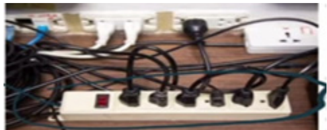
Fig. 3 Over Loading of Extension Board
